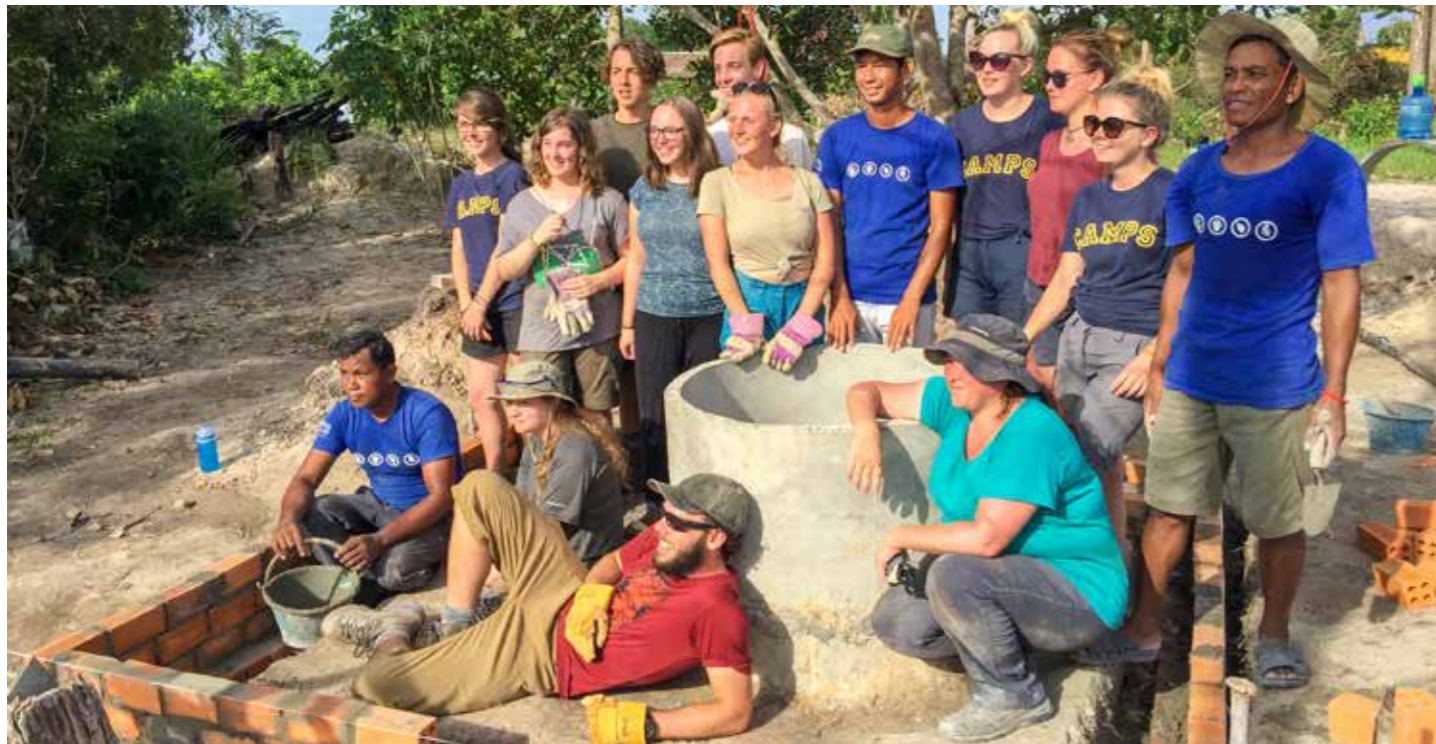
Top left: Preparing concrete well reinforcements. Top right: Lowering into place Above: Volunteers completing a well at Beng Pae
