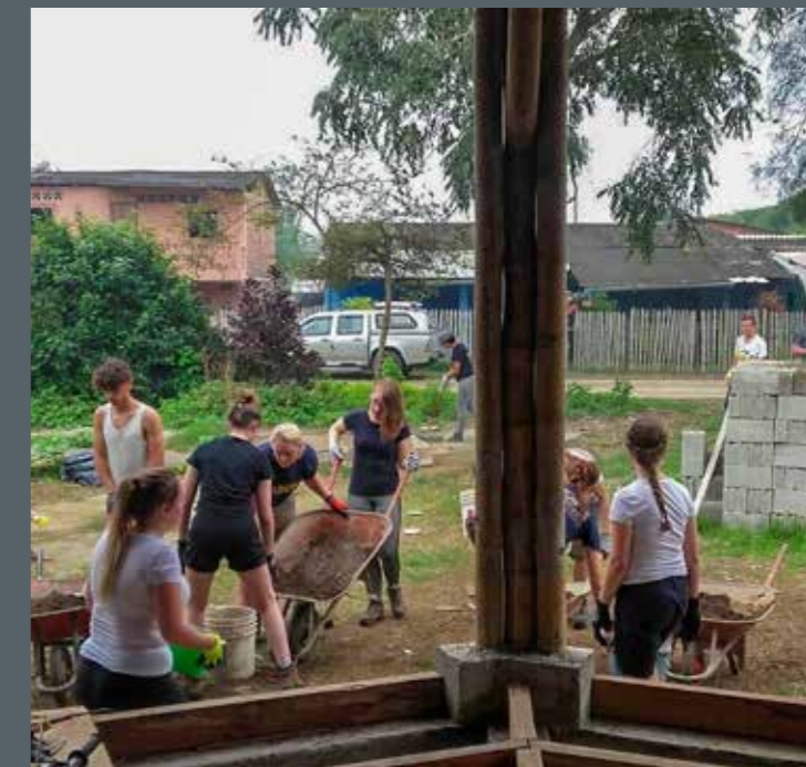
Above left: New playground at 26 Septiembre School. Above right: Refurbishing classrooms at Camilo Gallego School
