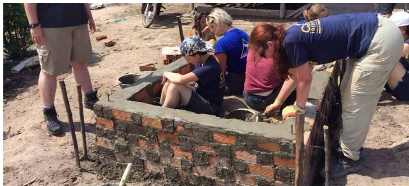
Top left: Concrete tube sections. Top right: Lowering into place Above: Building toilet walls at Beng Pae
