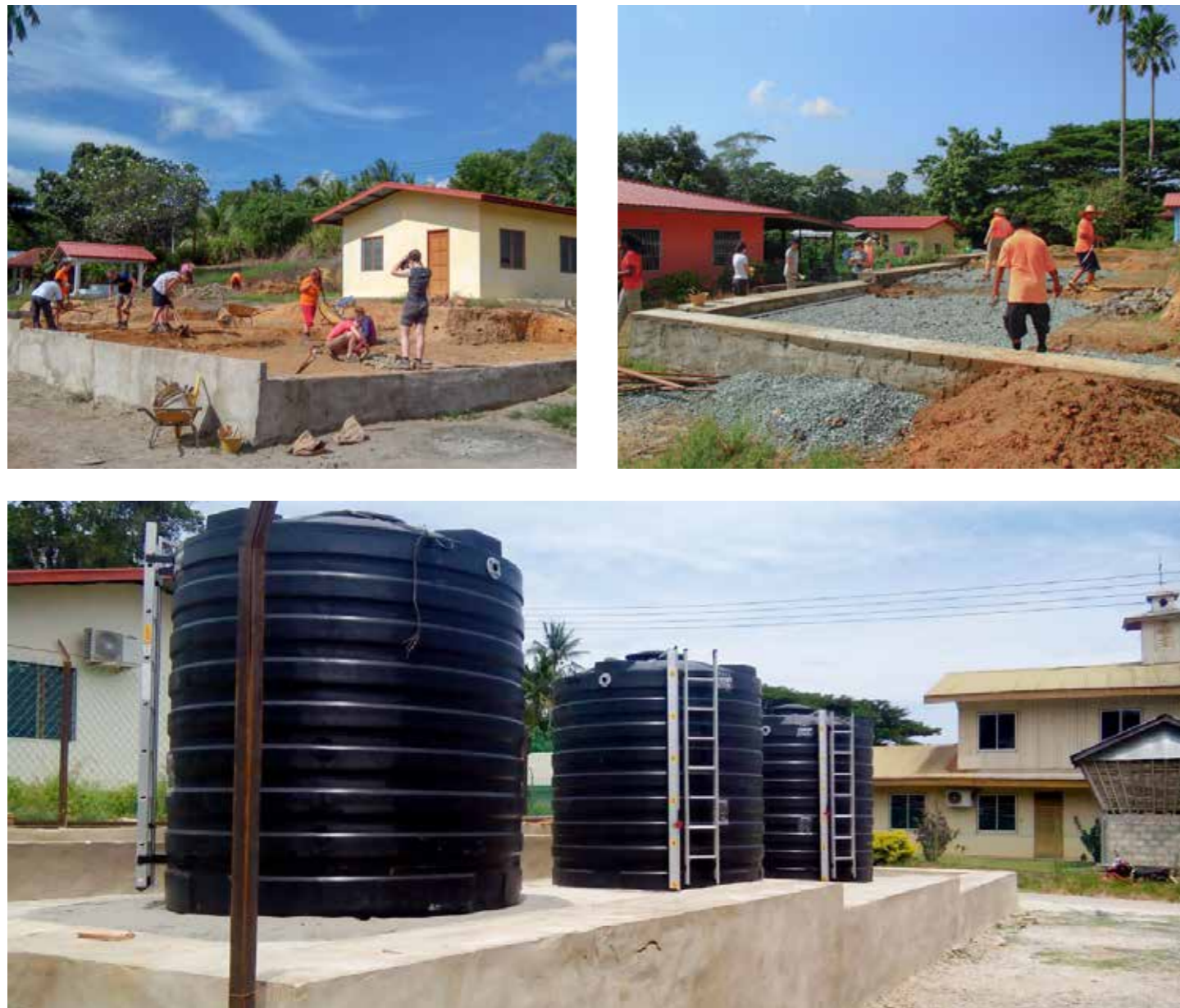
Top left: Levelling ground and building retaining wall. Top right: Laying foundations. Above: Final water storage system platforms
